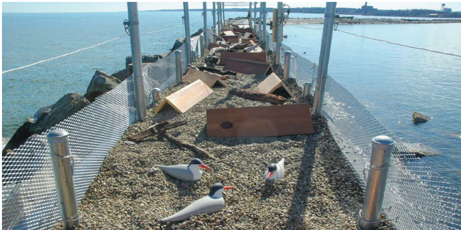
Armor stone repair of a breakwater in Ashtabula Harbor, OH. The project included creating nesting habitat at the top of the structure for the locally-threatened Common Tern.
